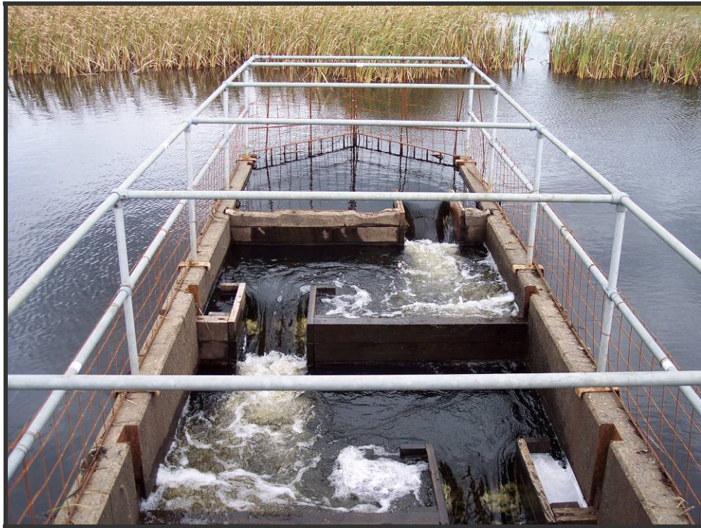
Figure 4 – Example of a Water Control Structure - Fish Baffles in Grand Falls–Windsor. Photo by: Charmaine Barney
