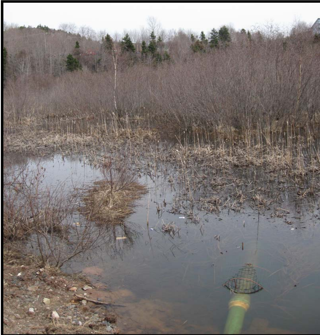
Figure 5 – Water Control Structure installed by Ducks Unlimited Canada at the Glynmill Inn Marsh, Corner Brook. Photo by Charmaine Barney
