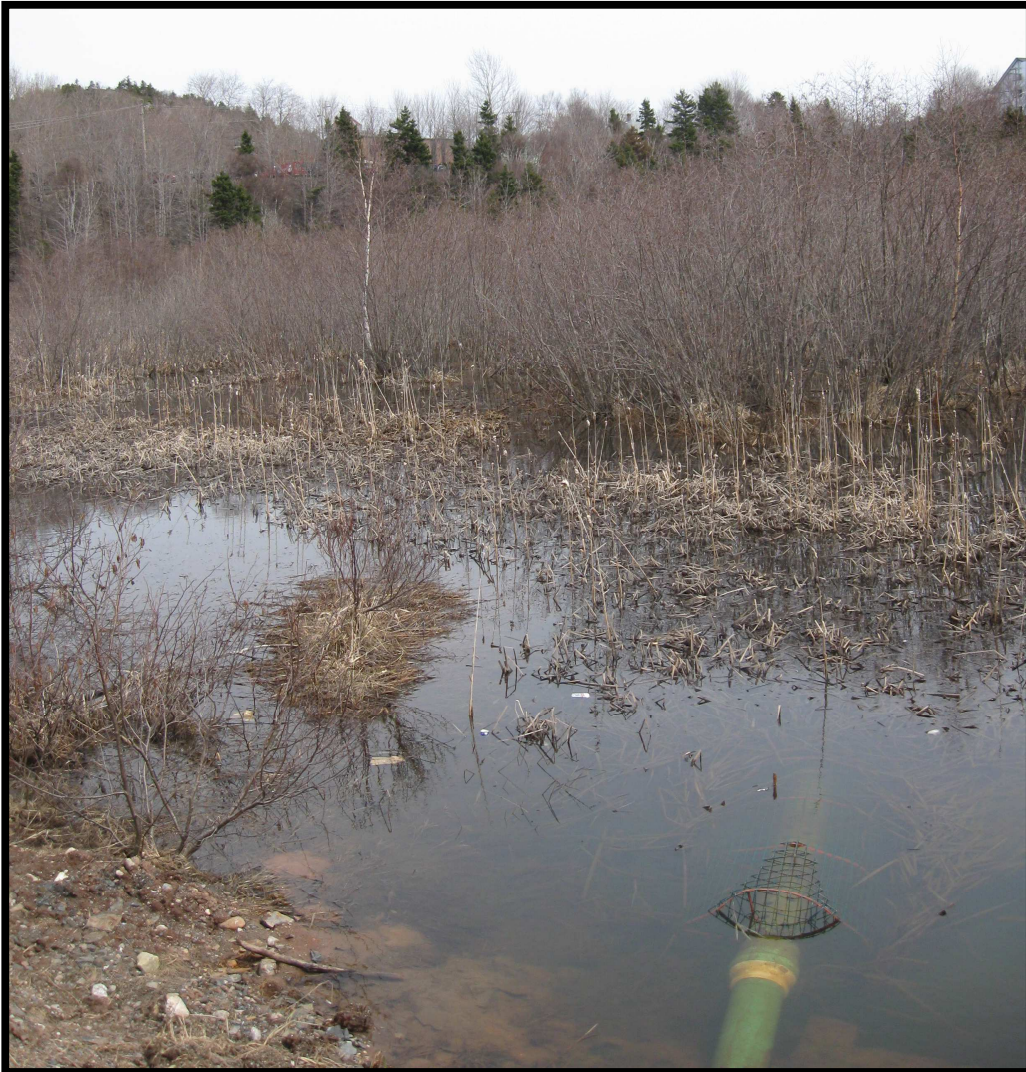
Figure 4 – Water Control Structure installed by Ducks Unlimited Canada at the Glynmill Inn Marsh, Corner Brook. Photo by Charmaine Barney
