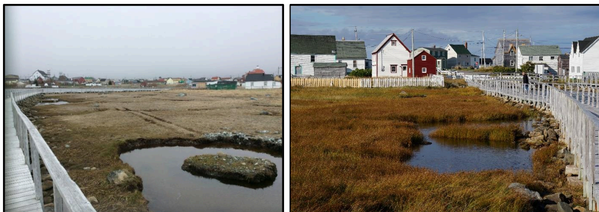
Lefthand photo: Construction in progress to dig out a former wetland and recreate islands; righthand photo: At the conclusion of the project - one of the completed islands showing new growth. Staff photos
