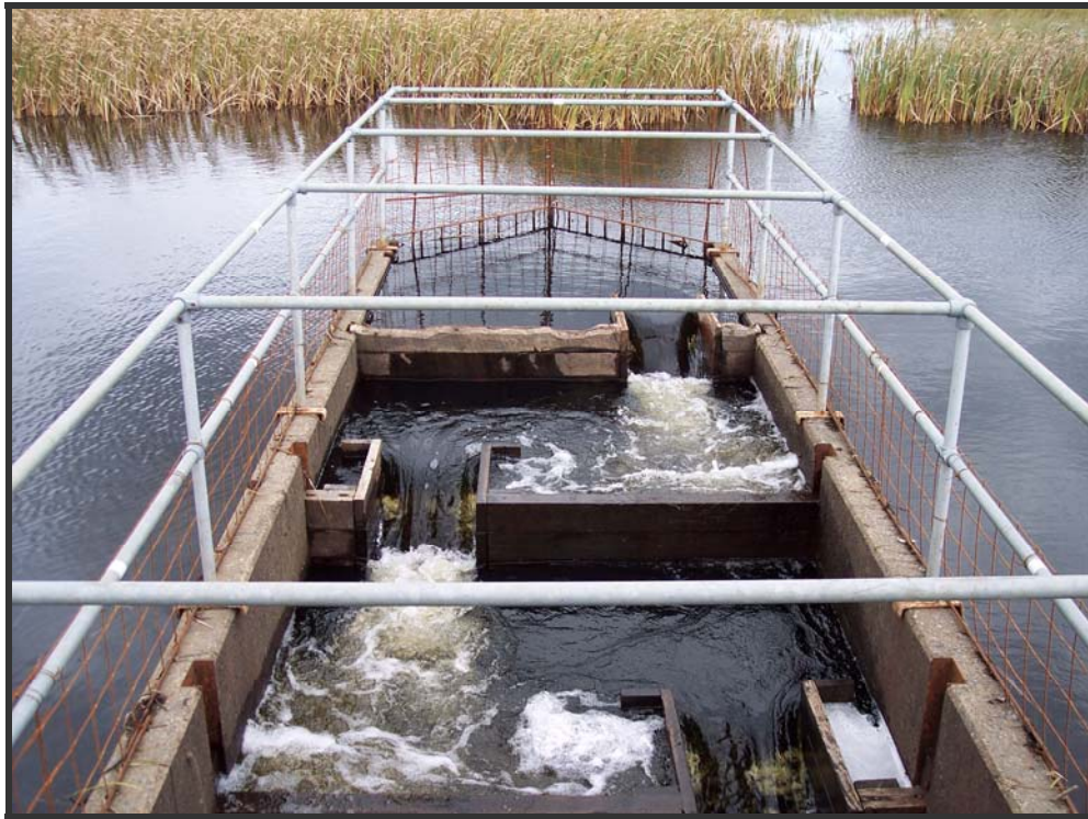
Figure 4 – Example of a Water Control Structure - Fish Baffles in Grand Falls– Windsor. Photo by: Charmaine Barney
