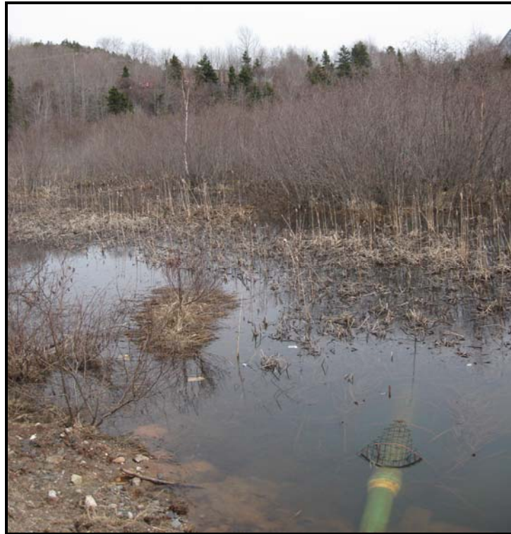
Figure 4 – Example of a Water Control Structure installed by Ducks Unlimited Canada at the Glynmill Inn Marsh, Corner Brook. Photo by Charmaine Barney
